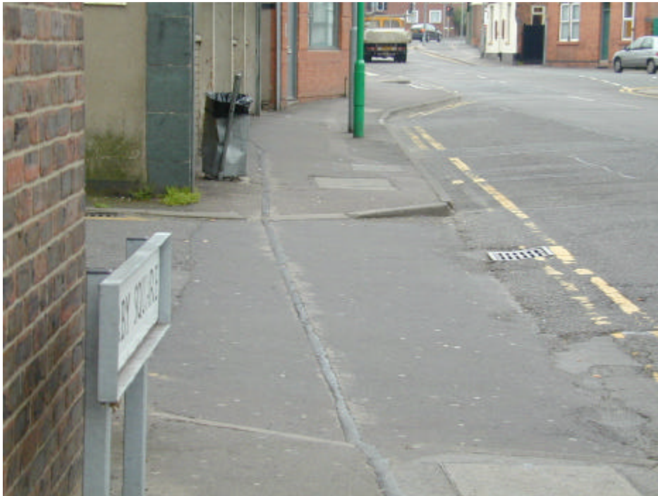
Figure 14: Narrow drop kerbs, uneven drop kerbs, litter bins and lamp posts.
